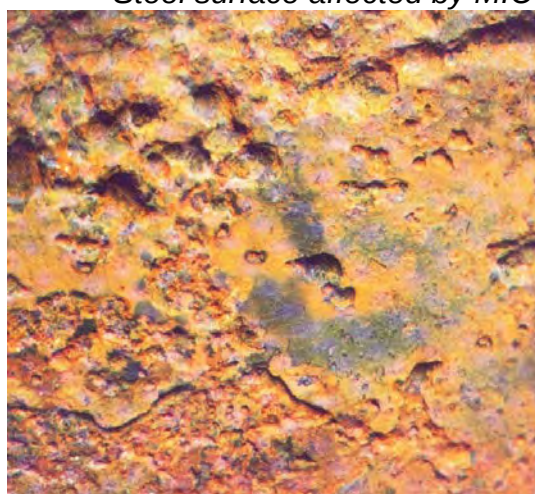
Steel surface affected by MIC
